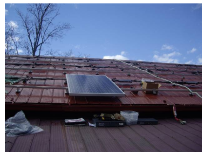
Installation on barn roof of John Cripton and Linda Sword
